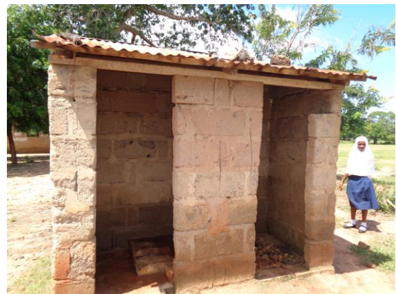
Permanent toilet facility in use for girls, that does not have doors, as noted in most of the schools
