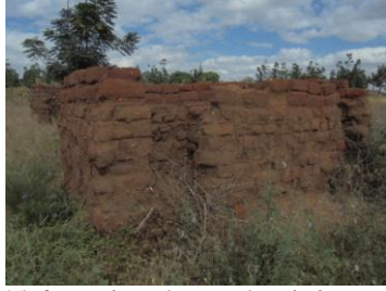
Toilets without doors and roof after two years ends from use
