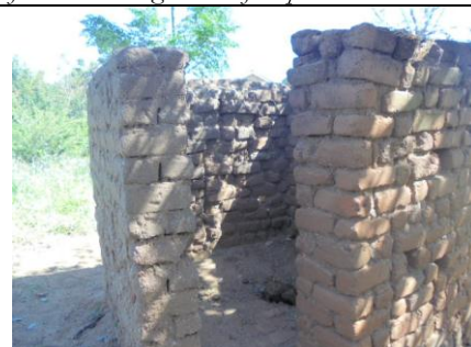
Toilets in most of the schools were found without doors and
