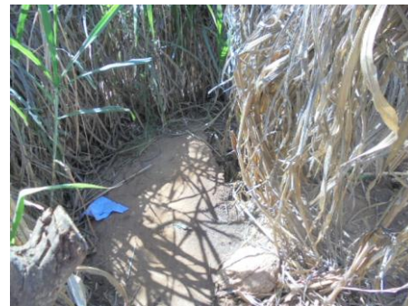
Toilet facility in one of the primary schools in Singida district, found in use regardless of its poor situation
