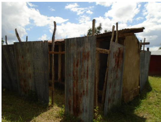
Permanent toilet facility in use for girls, that does not have doors, as noted in most of the schools
