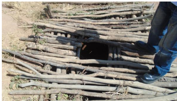
Very poor sanitation facility, and unsafe currently in use in one of the schools, as noted during baseline survey in Singida district.
